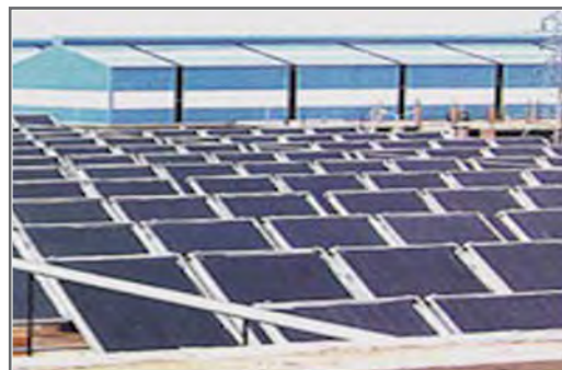
Fig 3.15: Solar Panels to trap solar energy
